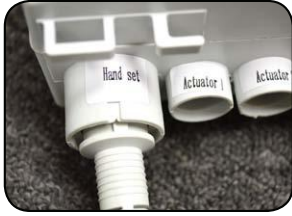
NOT Properly Inserted: The cord plug is flush with or sticking out of the outlet
