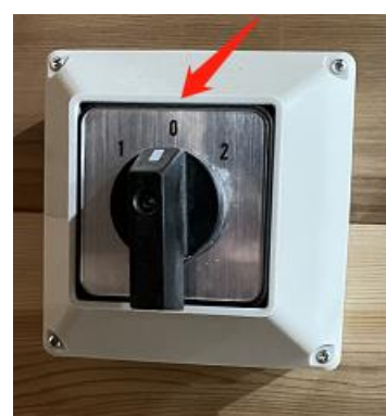
Power turned OFF
