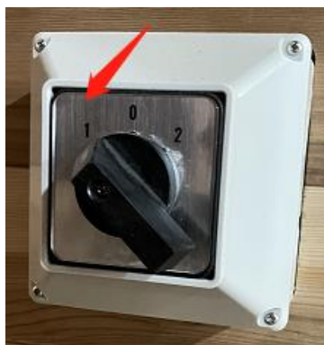
Power to stove heater
