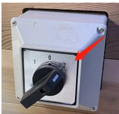
Power to Infrared heaters
