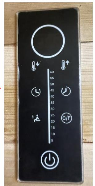
Sauna Control Panel has no Illumination
